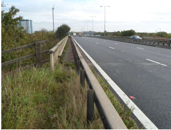
Figure 36 Discontinuous hard-shoulder at Langley Interchange
